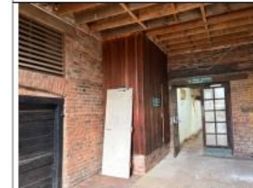
Potential asbestos in floor between Joists to be tested
